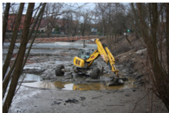
3.4 Dolní Břežany park Revitalization of lakes and stream in the central park
